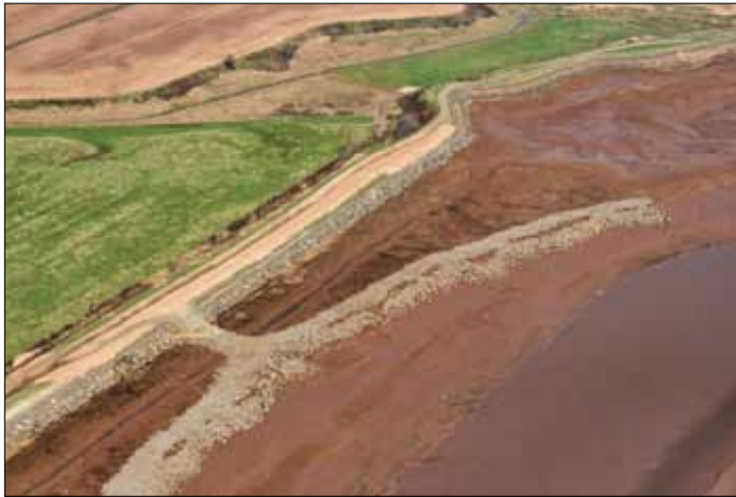
5-4 Breakwaters and rock facing on dykes mitigate the impact of storm surges.
